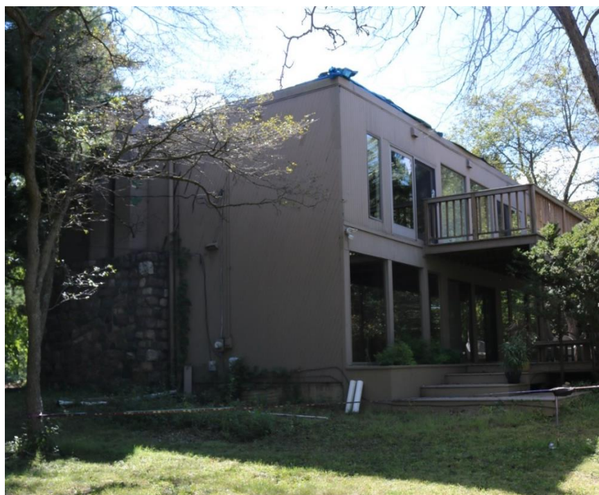
Rear elevation, note fire-damaged roof
