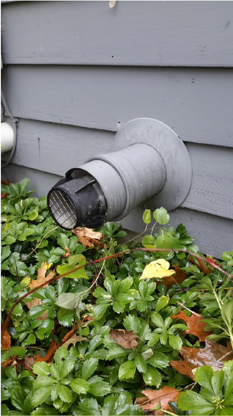
Example of PVC exhaust pipe; it will be painted brown to match the chimney
