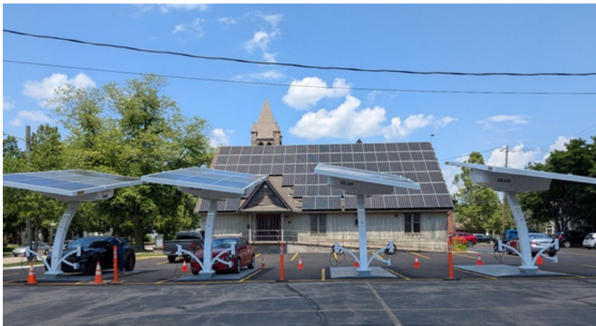
An installation of solar paneled EV chargers at the Ypsi Performing Space at 218 N Adams St. expands the public EV charging network throughout the county
